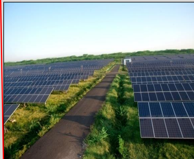
5 MW Solar Plant at SLPP (2012)
