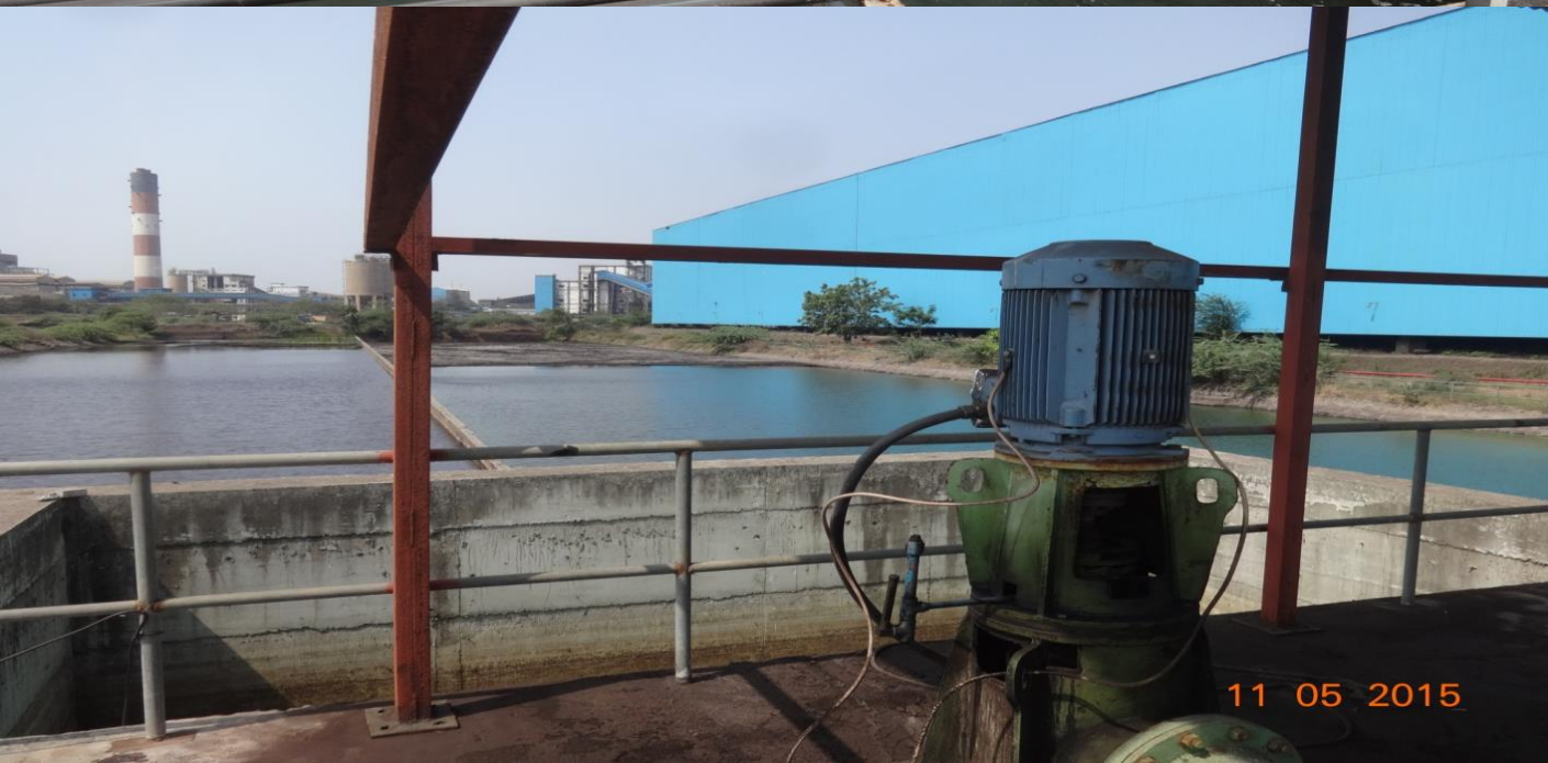
Run-off Pond Water Transfer Pumping Station
